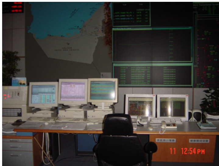
Fig. 1 Power System Control Center
